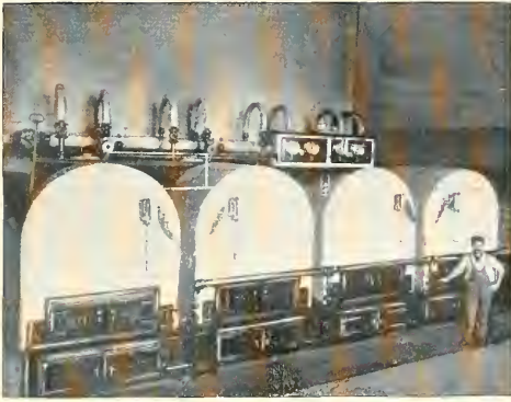
Boiler Room—Warren Hospital.
